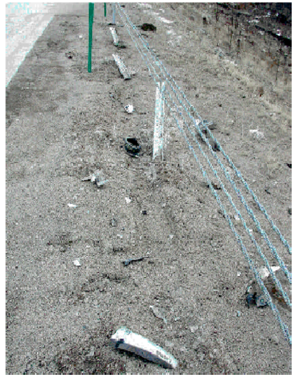
Brifen Guardrail After Accident
